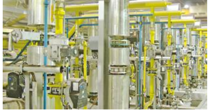
Walking beam furnace with overhead firing
