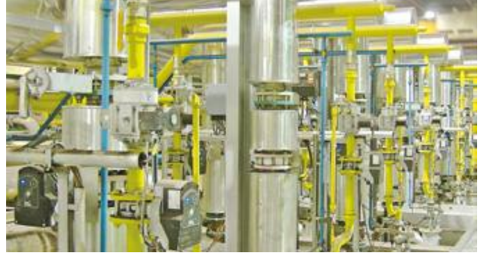
Walking beam furnace with overhead firing
