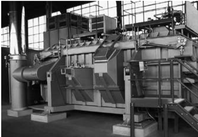
Aluminium industry: smelting furnace
